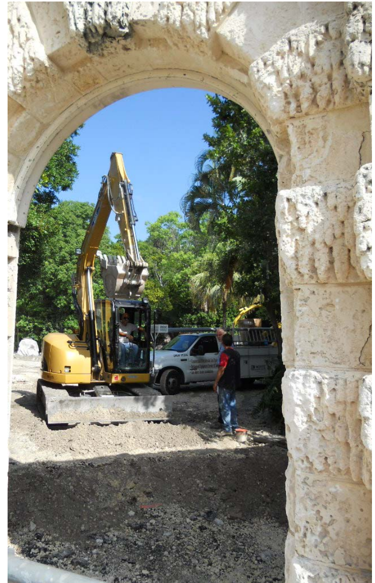
Construction crew reconstructs the service road, below which the stormwater pump/pollution filtration system is located.
